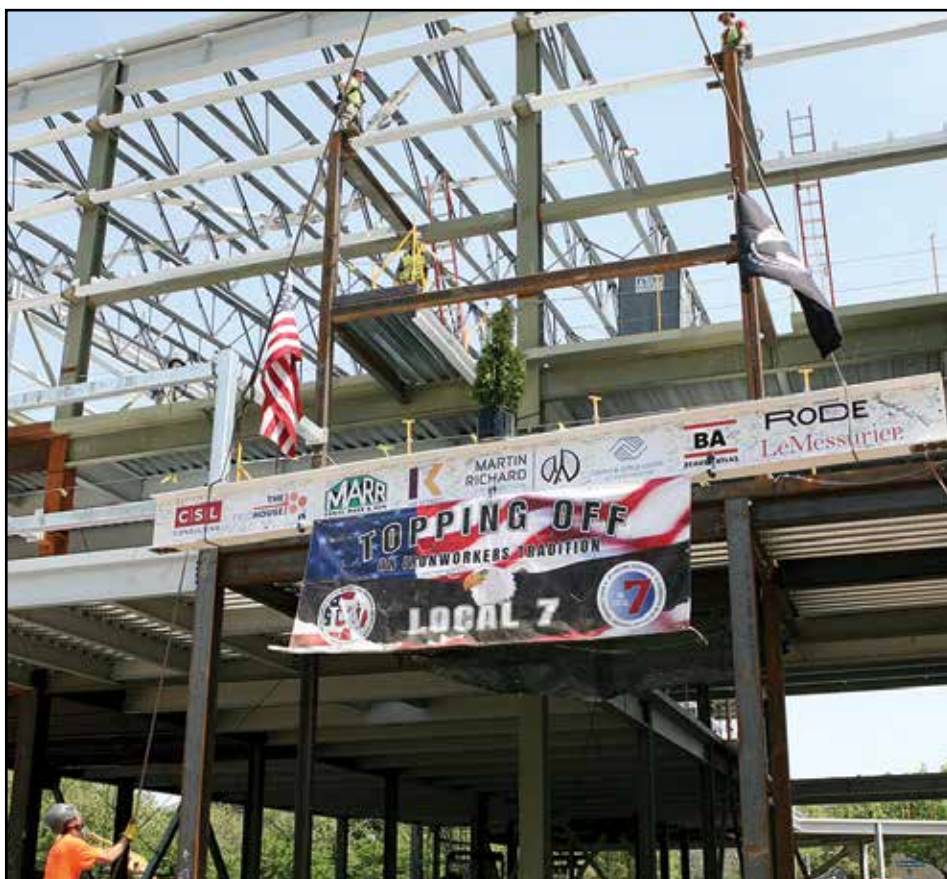
The ceremonial last steel beam was lifted into place for the "topping off" on the Fieldhouse+ project on Mt. Vernon Street on Monday (May 18).
